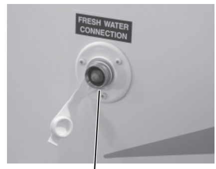
City water connection - note filter screen.
